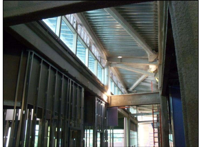
Figure 18 - Shown above is the clerestory that stretches over 200 feet long and bringing in natural light. Personal photograph taken by Chris Pozza.
