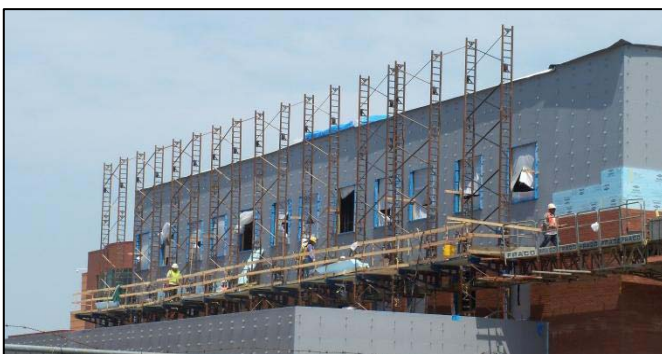
Figure 14 - View looking at southwest elevation. A MasonKing lift is required in areas where work is done above rooftops. These lifts have to be simultaneously cranked by hand on each side to be lowered or raised. Personal photograph taken by Chris Pozza.
