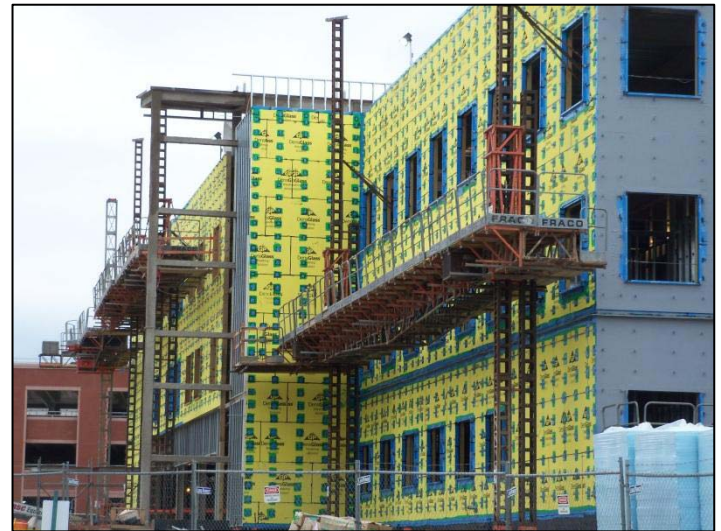
Figure 47 - View looking at the corner of the south and east façade. DensGlass can be seen in yellow, with each individual brick tie having Blueskin applied. This is a necessary step before the air and vapor barrier can be applied. Personal photograph taken by Chris Pozza.
