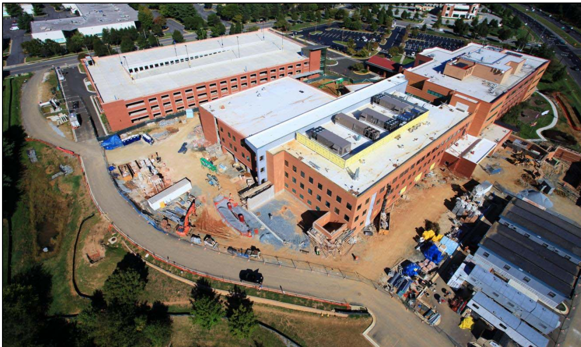
Figure 1 - Progress photo of the addition taken in September 2012. Image courtesy of DPR.
