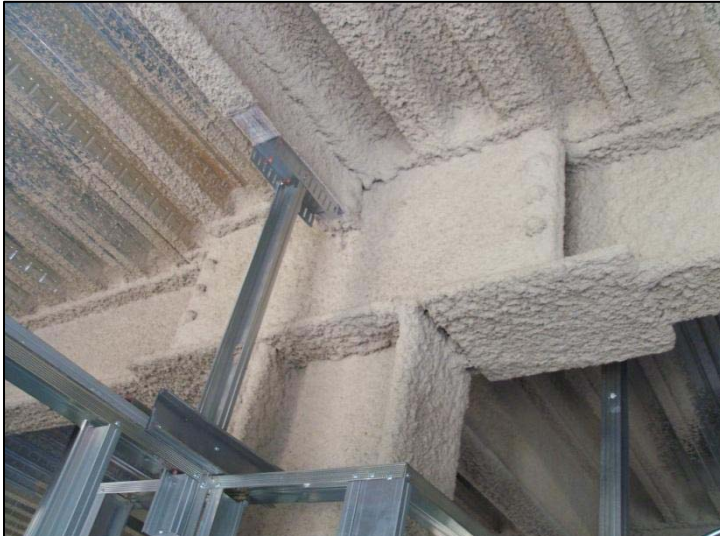
Figure 6 – Photograph of a SidePlate system which is a moment frame that connects columns to beams and girders and can be a single- or double-sided connection. Spray-on fireproofing has already been applied to the structural steel at this point of construction. Personal photograph taken by Chris Pozza.
