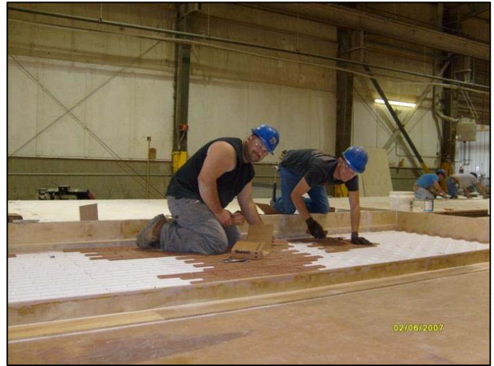
Figure 37 - Workers are able to fabricate panels comfortably in a controlled environment; increasing quality and productivity. Image taken from Gate Precast.
