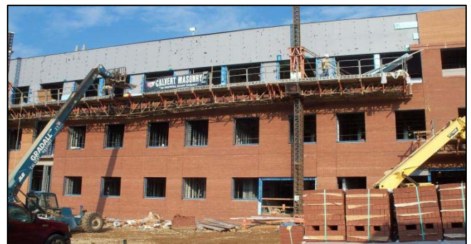
Figure 15 - View looking at east elevation. Fraco Lifts are used around the exterior to provide an efficient workflow along a large percentage of elevation at a time. Materials are lifted into place with a boom lift. Personal photograph taken by Chris Pozza.
