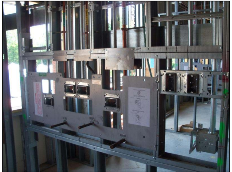
Figure 61 - Headwall template can be seen in place with medical gas and conduit rough-ins. Personal photograph taken by Chris Pozza.
